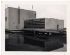
Air Conditioning Tower on the Courthouse Roof (100-03-01-0406)
