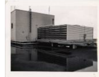
Air Conditioning Tower on the Courthouse Roof (100-03-01-0406)
