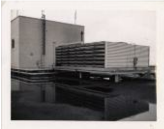
Air Conditioning Tower on the Courthouse Roof (100-03-01-0406)
