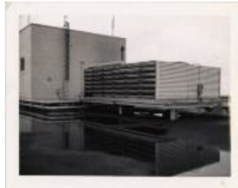
Air Conditioning Tower on the Courthouse Roof (100-03-01-0406)
