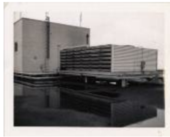
Air Conditioning Tower on the Courthouse Roof (100-03-01-0406)
